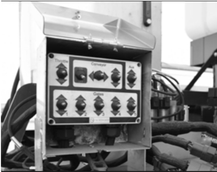
Fig. # 4-25 Hydraulic Hopper Gate Controls
